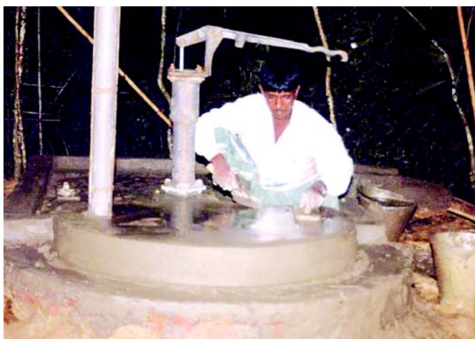
Construction of a dug-well in Bangladesh which uses a shallower aquifer to provide "arsenic free" water.
